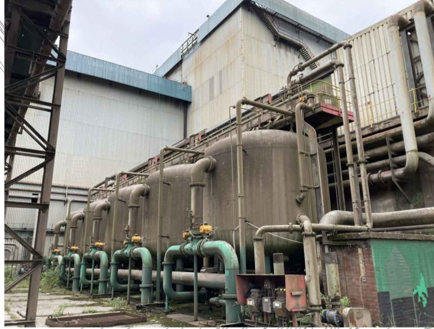
SAND FILTERS AND PUMPHOUSE
